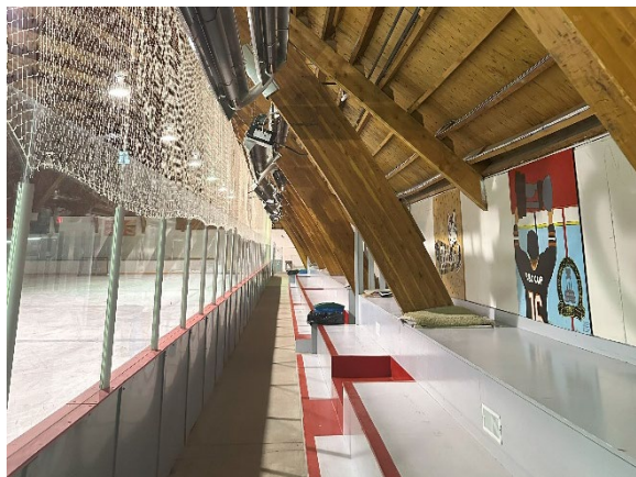
Figure 31: Gas Tube Heaters over Spectator Seating
