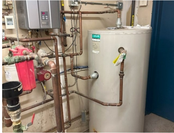
Figure 52: Hot Water Tank
