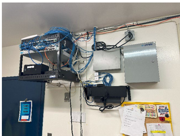
Figure 39: Arena Office Wiring
