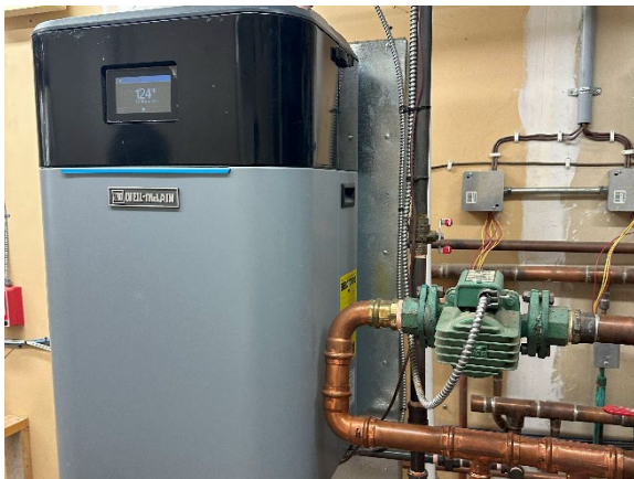
Figure 53: Hot Water Tank
