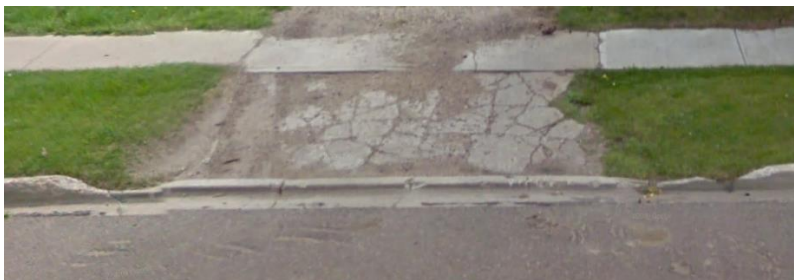
Straight face curb, or curb broken off – must be replaced.
